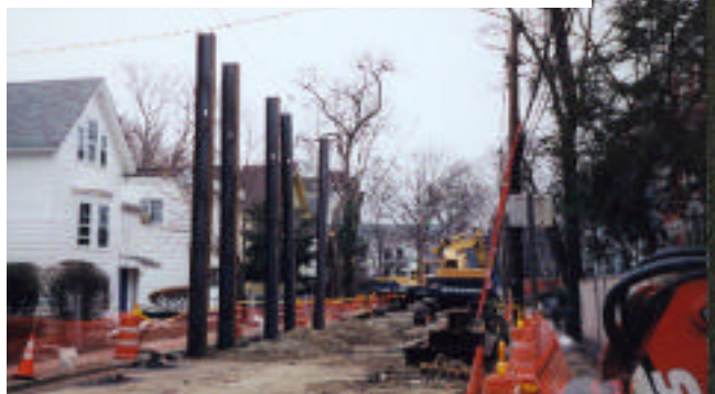
February 2001, Wendell Street-vibrating in the 25 foot beams that shore up the excavation
